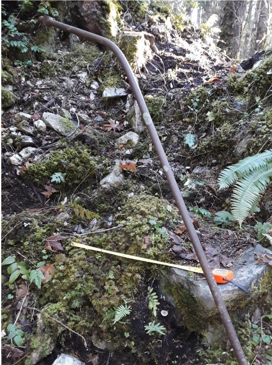
Figure 15. Metal bar on north side of kiln structure. Metal bars were installed around the masonry bases of lime kilns to add structural integrity.
