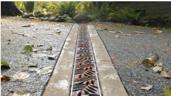
Grates allow stormwater to pass through while allowing for pedestrian movements.
