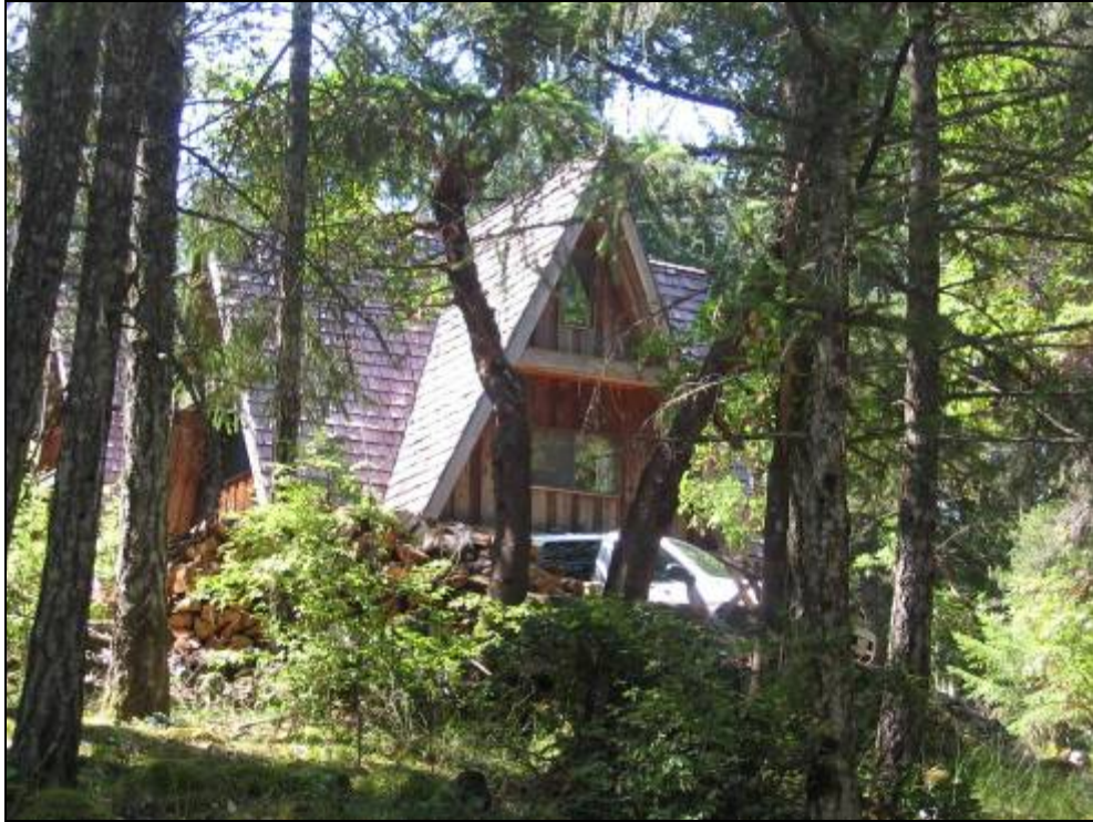
Figure 12. Photograph showing unrated roofing material present on some homes within the wildland urban interface.
