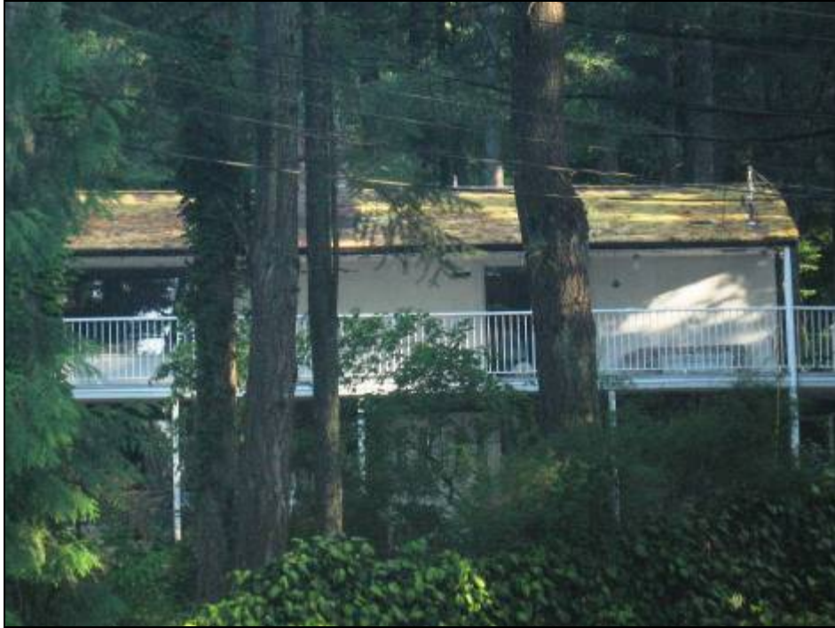
Figure 14. Example of a home with open deck, no setback to forest vegetation and roofing with debris capable of igniting due to ember showers.
