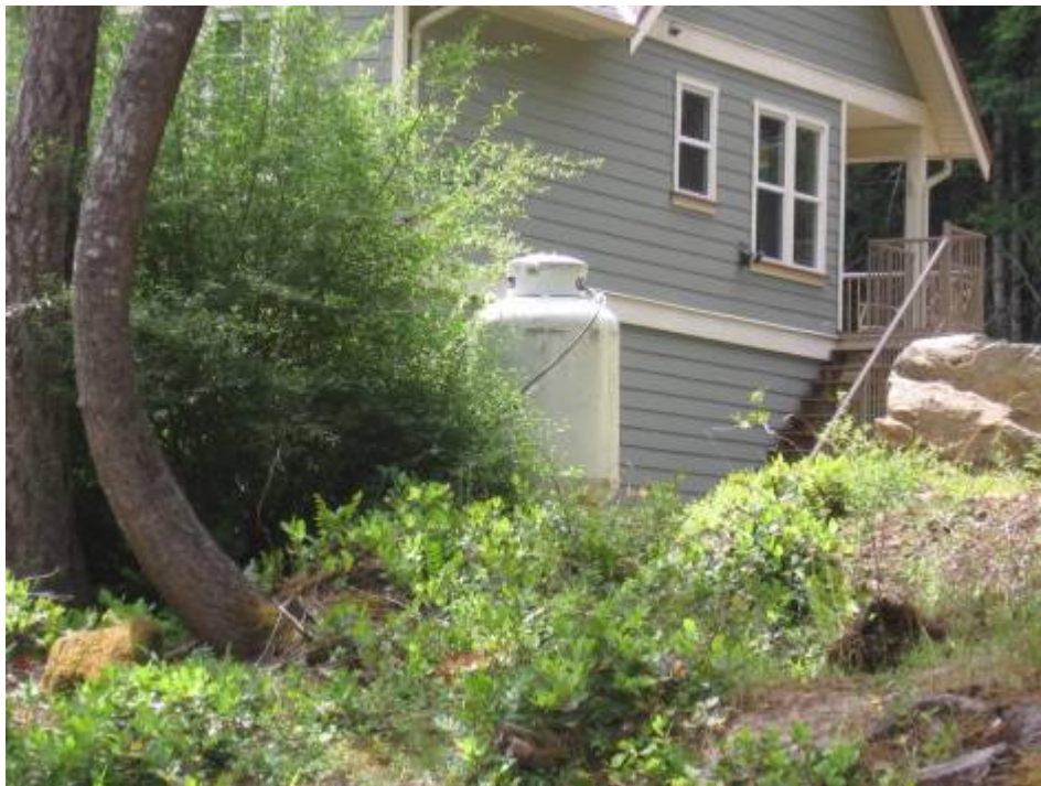
Figure 15. Propane tank close to residence and vegetation.
