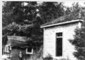
Deteriorated School House & Teacherage
